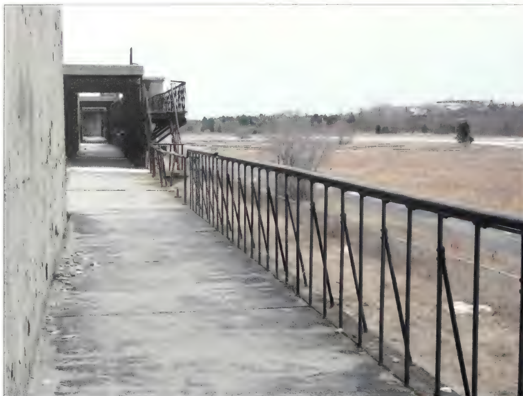
Figure 3.19. View looking south at existing guardrail, Nine Gun Battery. Both handrails and guardrails are present at Nine Gun Battery and are generally in good to fair condition (Olmsted Center, January 2009).
